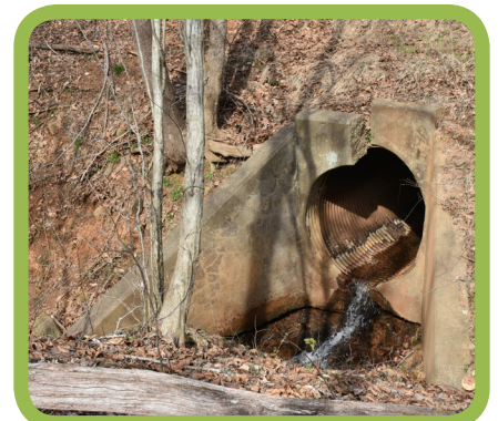
An existing stormwater outfall from Interstate 64 near the Old Mills Trail. This type of facility is discouraged.
