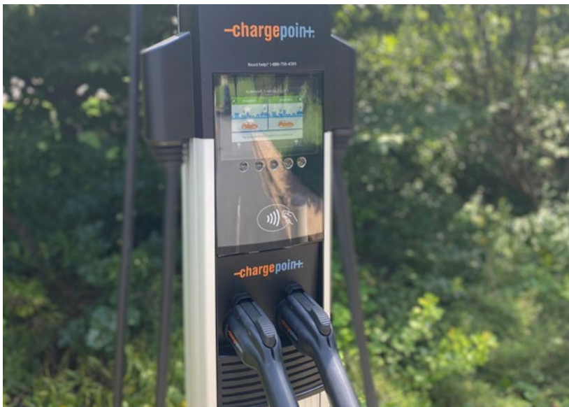
Electric vehicle charging station at the Albemarle County Office Building on McIntire Road.
