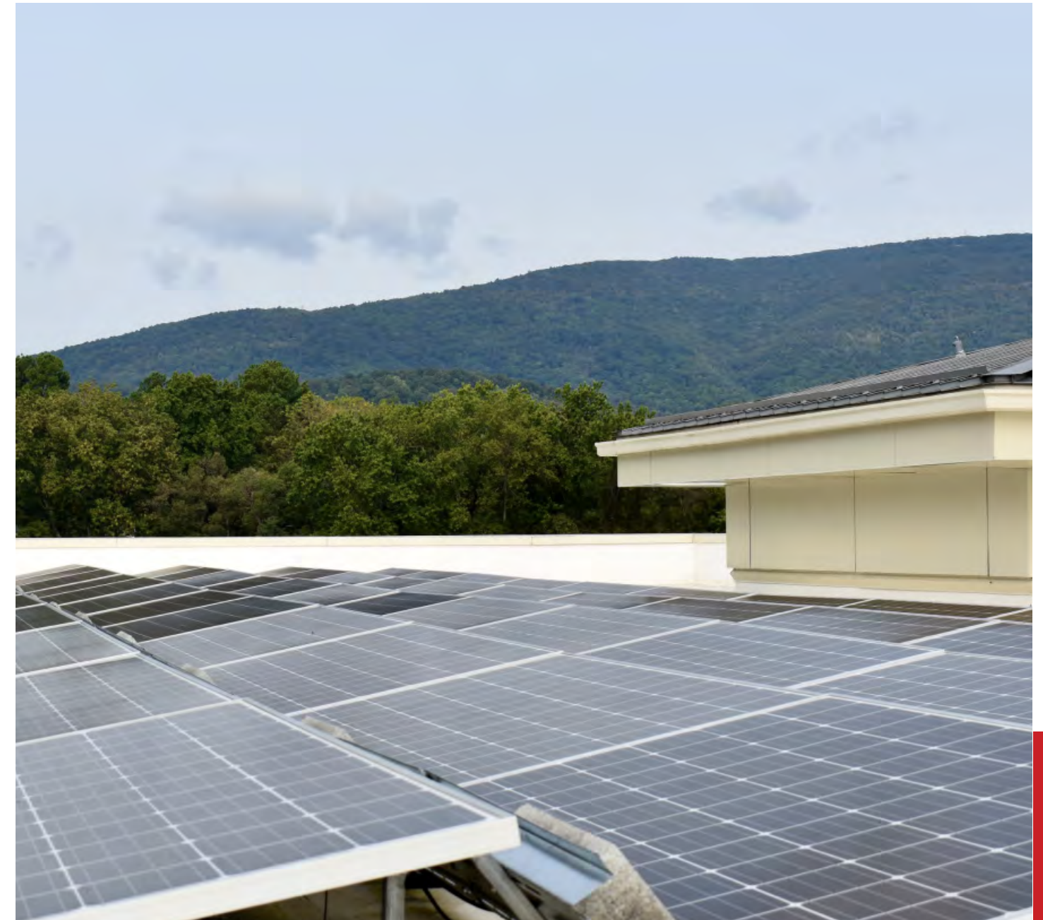
(Above) Solar panels on the Crozet Library.
